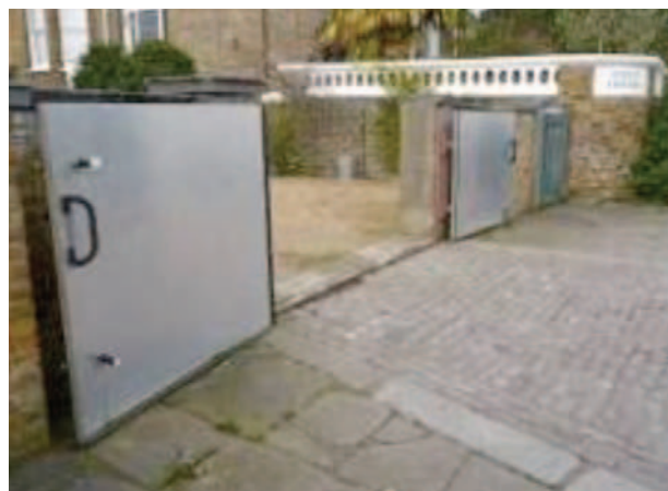
Above: Example of a flood gate installed to a communal car parking area
