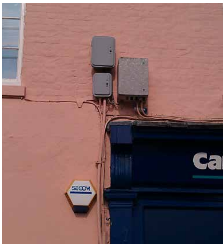
Alarm boxes should be as discreet as possible
