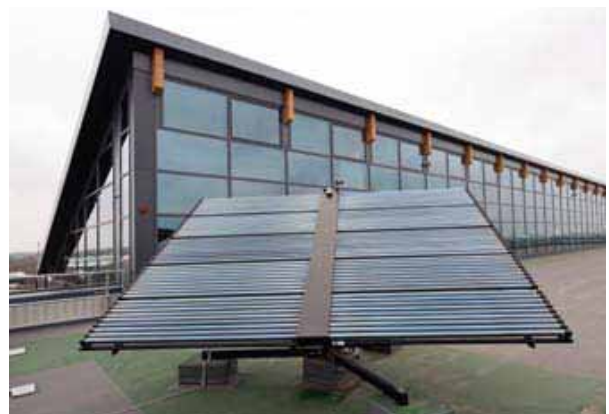
Solar hot water collector
