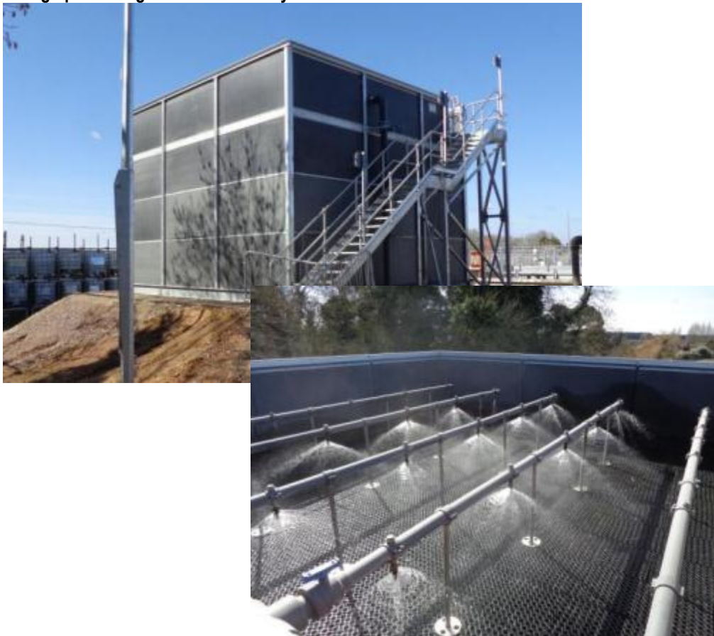
Photograph 5 Cougar Bio-Blok Tertiary Filter
