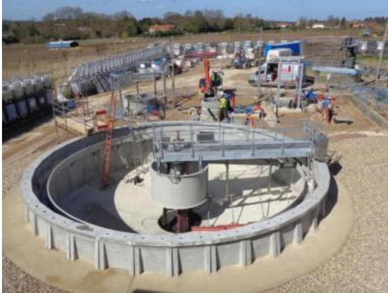
Photograph 6 New Final Settlement Tank
