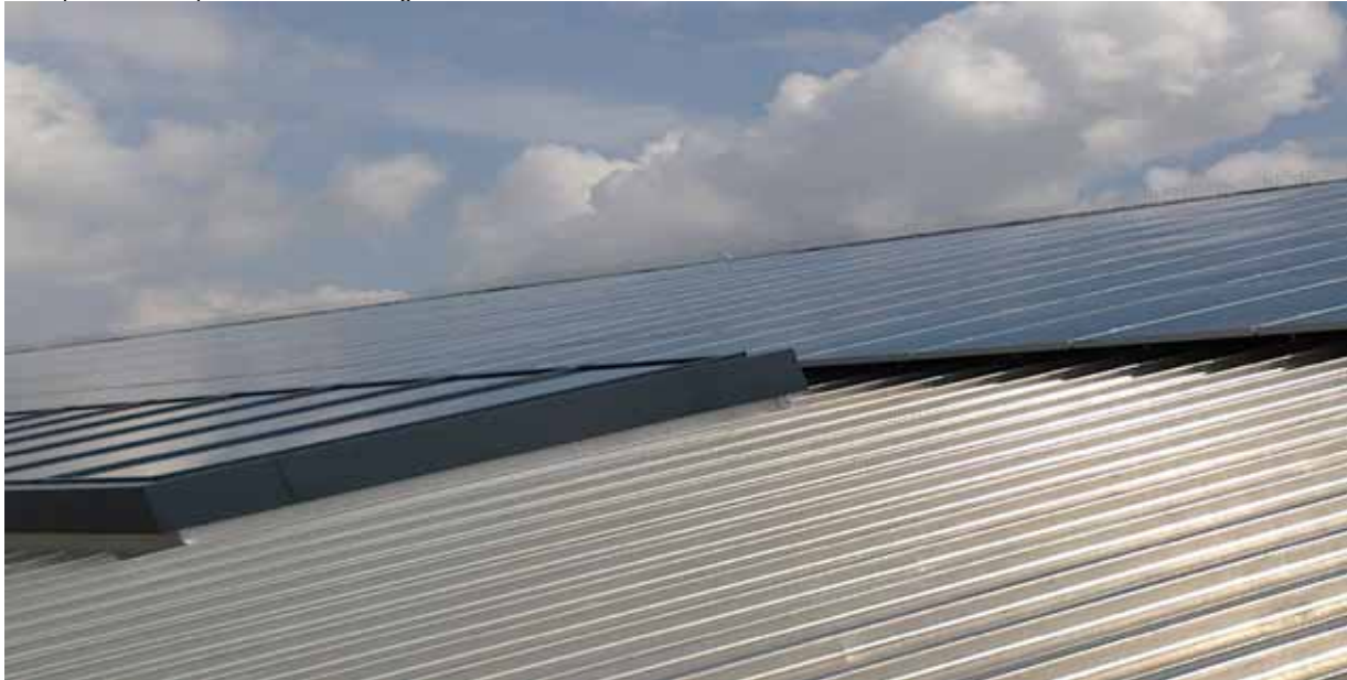
Solar photovoltaic panels above roof lights, West Suffolk House
